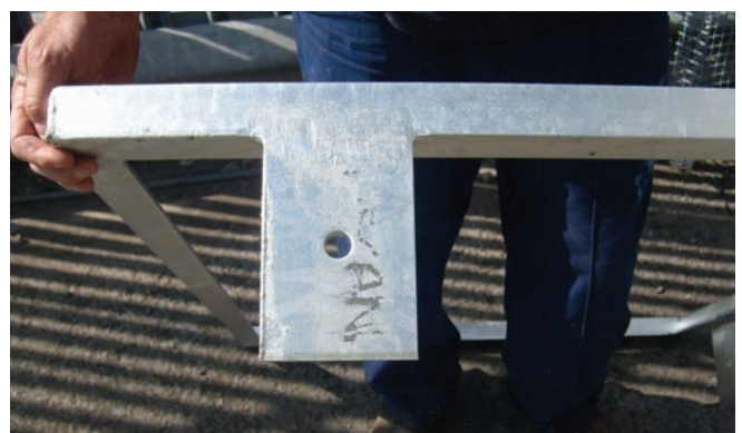
Three examples of bare steel where customers or their suppliers have written on the steel with crayon, paint or solvent based markers. This bare steel is prone to corrosion.
